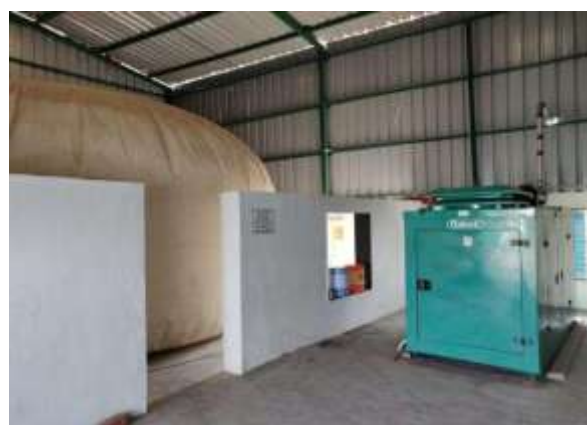
Biogas storage and generator
