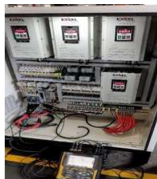
Fig. 2.2 PQA Meter Installation
