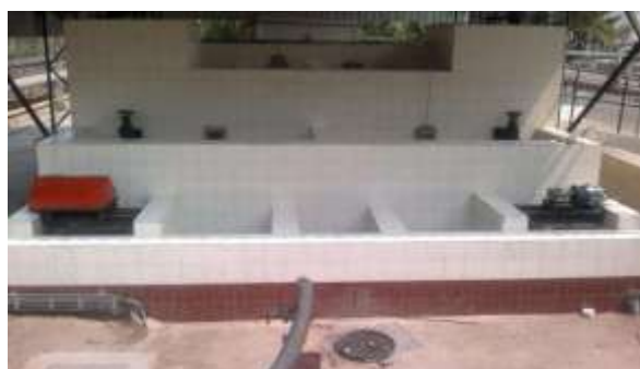
Crushing/Mixing Unit with Inlet Chamber
