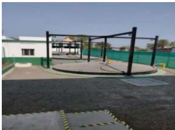
Gas Generation System
