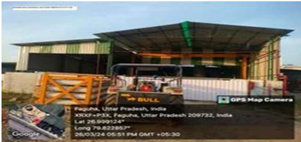
Fig-1 Generator with Gas Engine
