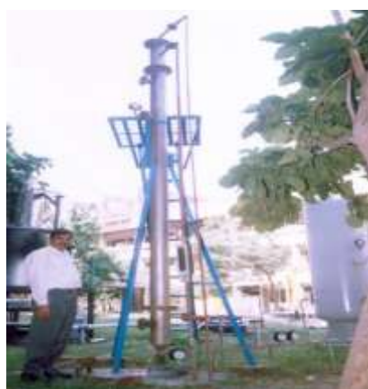
Plate-1: Scrubber for purification of biogas
