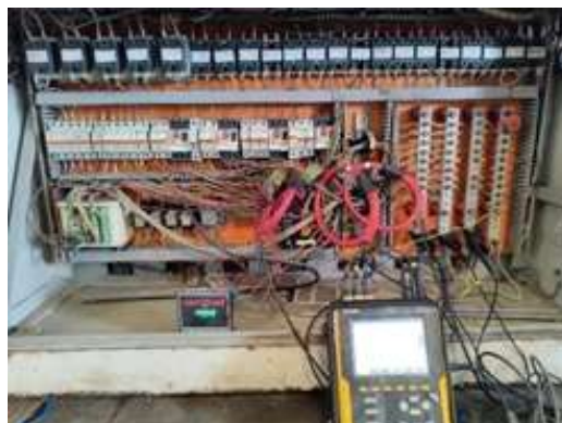
Fig-2.12 PQA Meter Installation
