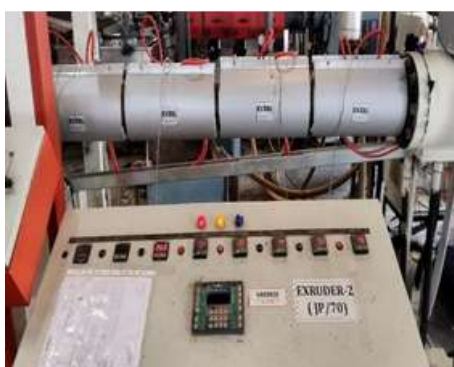
Fig-2.1 Existing Induction Heater
