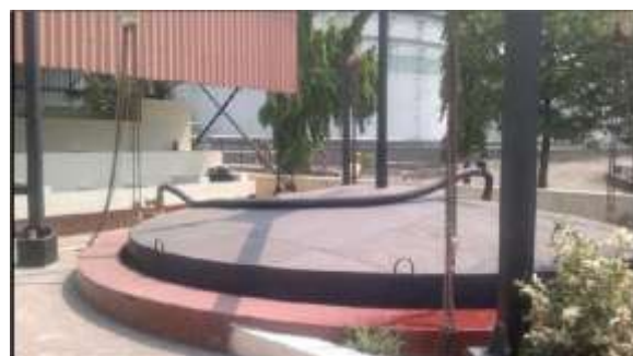
Digester and Gas Holder Tank with outlet Pipe
